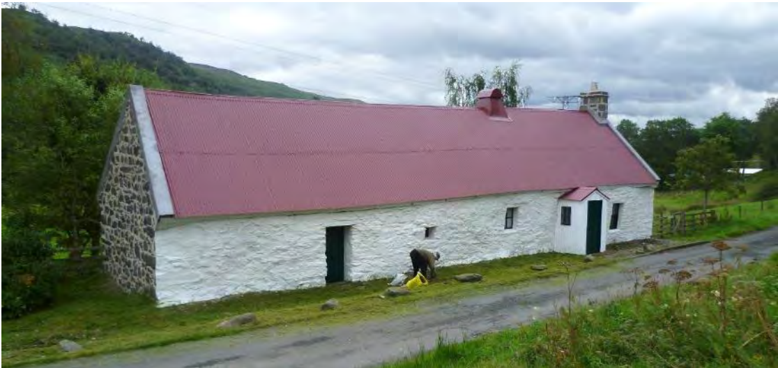
Fig. 7: Moirlanich Longhouse, weak earth mortared rubble with lime pointing & wash. The leaning section to the right of the porch is shown in repair below.
