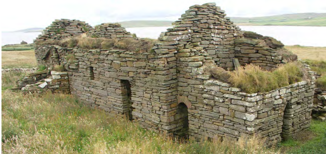
Fig. 23: Eynhallow Monastery, Orkney, movement of masonry followed erosion of earth mortar.
