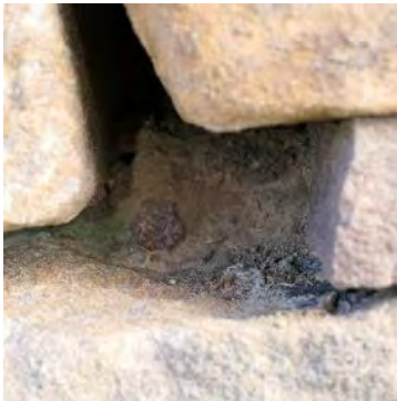
Fig. 18: Earth mortar, severe external decay.
