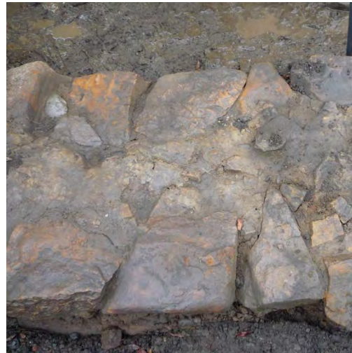
Fig. 14: Earth mortar, note no lime.
