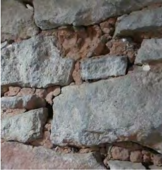
Fig. 5: Example of earth mortar, used as dug, from very close to site, Main St. Longforgan, early 19th C. Shrinkage cracks as a result of high clay content in chimney wall.
