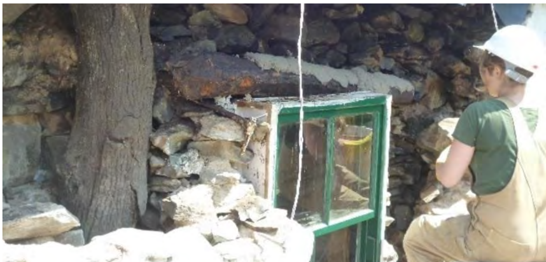
Fig. 8: Back face of inner leaf exposed during repairs at Moirlanich, with cruck leg having benefitted from the preserving effect of earth mortar drawing away moisture.
