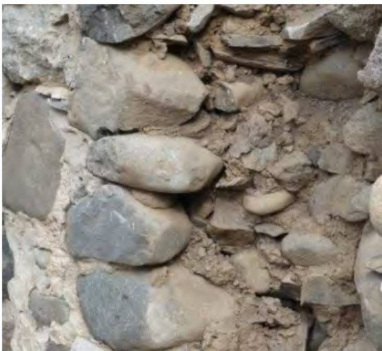
Fig. 21: Earth-mortared wall with lime pointing, the face having fallen away due to water ingress at the wallhead and lack of restraining through stones tying the outer to the inner face.
